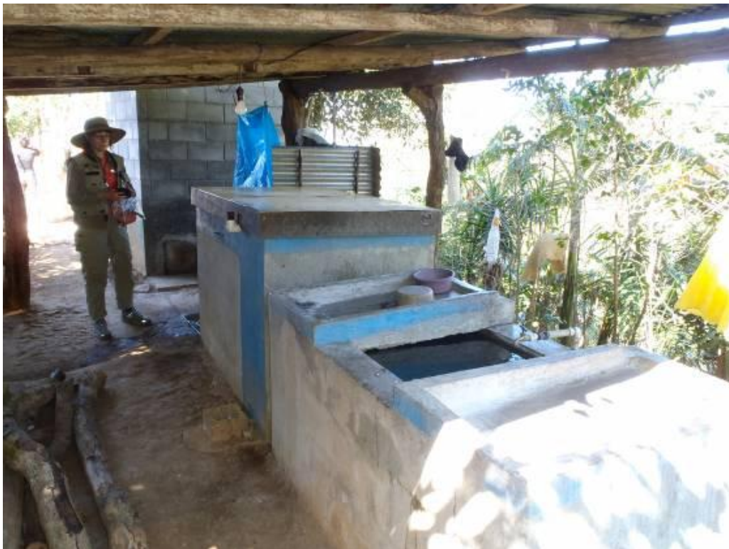
Figure 2.2.2 Water storage tank connected to the infiltration gallery in Las Mercedes
