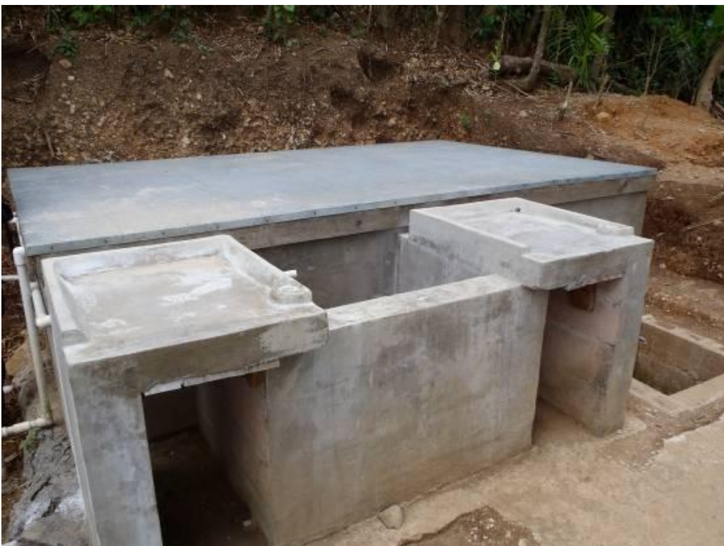
Figure 2.2.6 Water storage tank connected to the infiltration gallery
