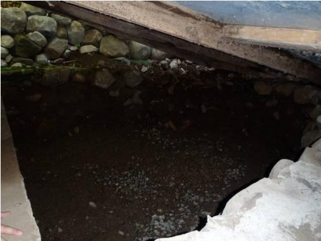
Figure 2.2.5 Inside the infiltration gallery in La Cumbre
