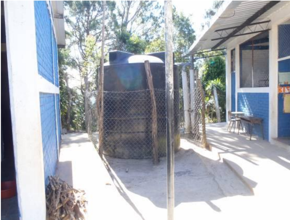
Figure 2.2.1 Rainwater catchment tank at the El Naranjito School
